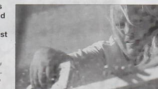
Clark with a staple gun to build a float. // JERRY TING // MOSAIC STAFF
